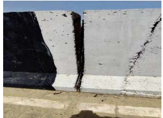
ROB at CH 8+954
