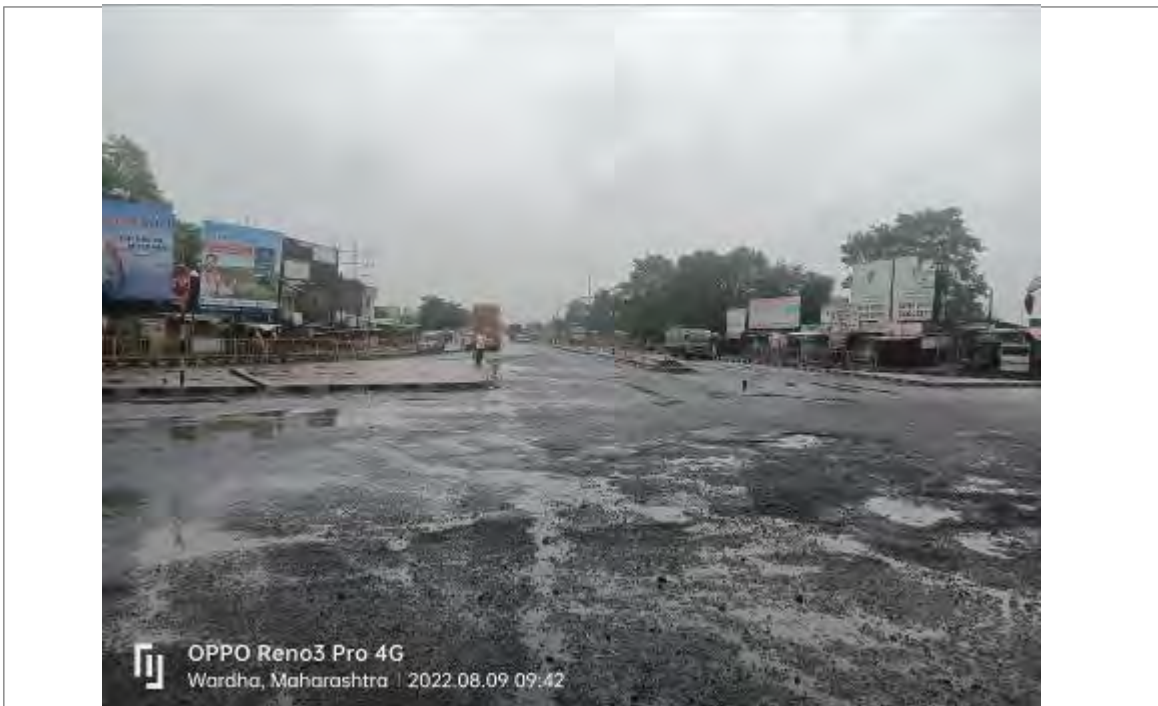
Photo 4: Potholes on the highway
