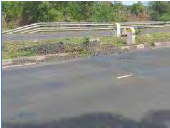
Pothole at Km 143.300 LHS
