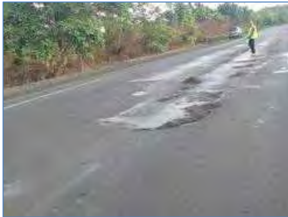
Bleeding & Patching at Km 127.700 RHS
