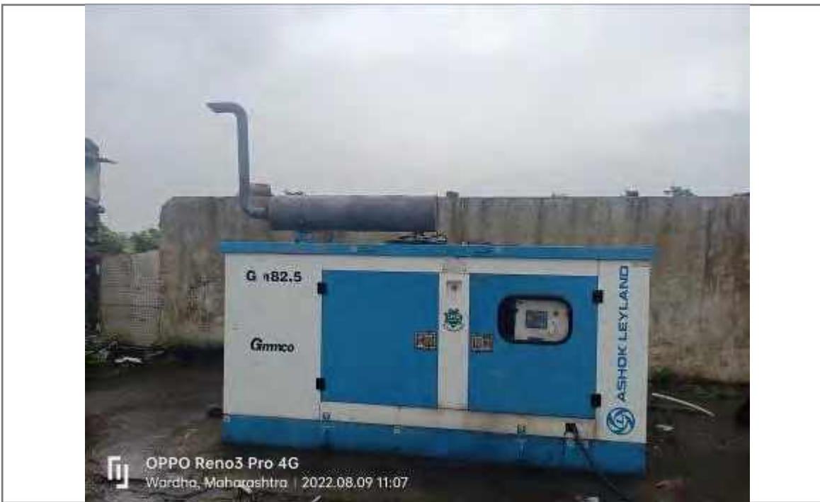
Photo 11: Diesel Generator at the toll plaza
