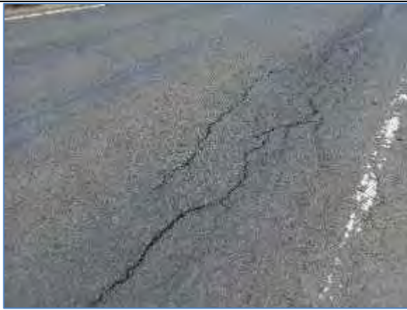
Longitudinal cracking at Km 59.100 RHS
