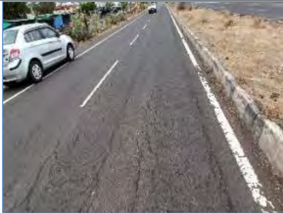
Rutting at Km 113.600 RHS
