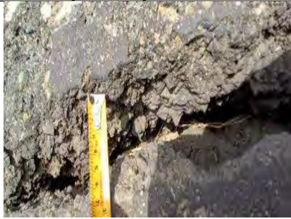
Cracking at Km 44.300 RHS
