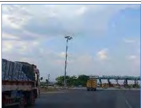
High mast lighting at Junction near Km 95+570 RHS
