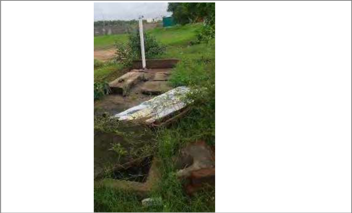
Photo 11: Septic tank in the toll plaza premise
