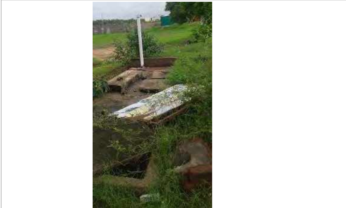
Photo 11: Septic tank in the toll plaza premise
