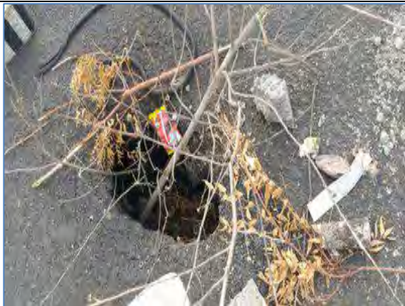
Pothole at Km 43.200 RHS
