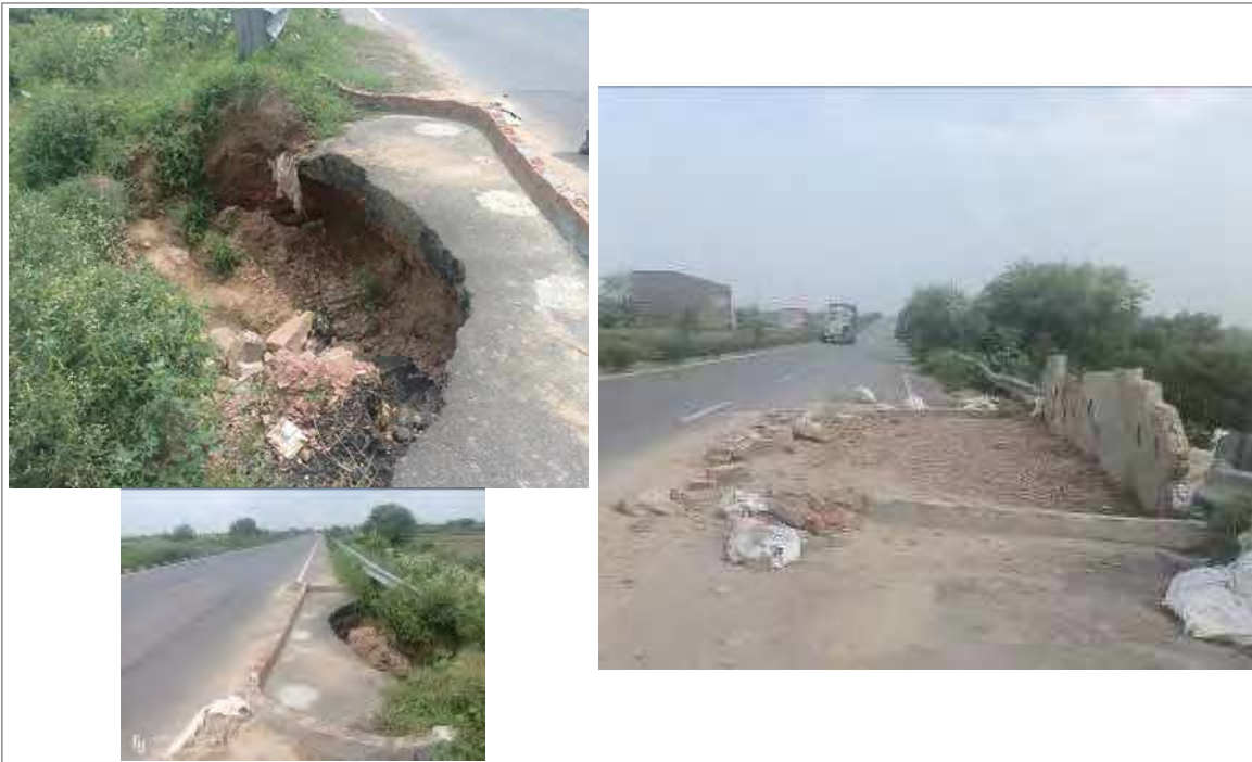
Photo 4: Road subsidence along the National Highway
