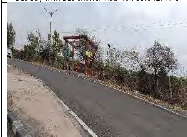
Damaged bus Shelter at km 127.585 LHS
