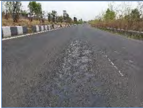
Bleeding at km 92.000-LHS
