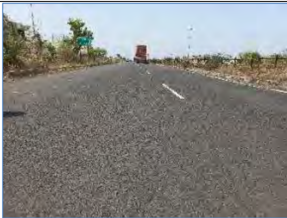
Raveling at km 95.300-LHS
