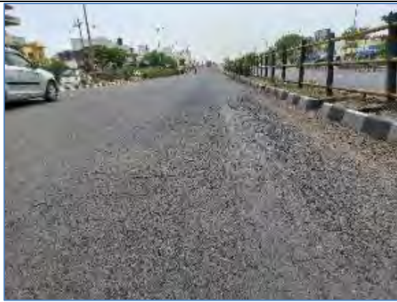
Alligator cracking at km 74.900-RHS
