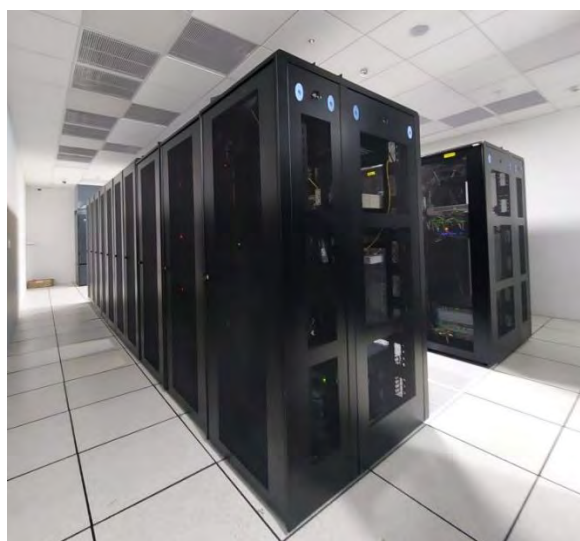
Fig 6.1 KFON ISP Room Network Rack
